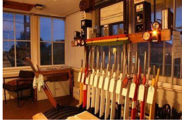
Shippea Hill signal box interior. Same style as Lakenheath box.
